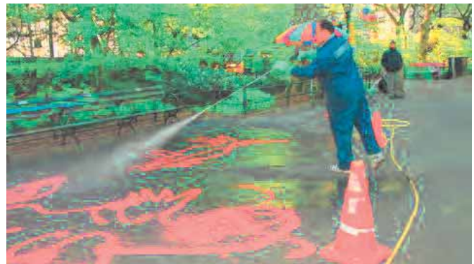
Figure 2.4. Graffiti removal may require temporarily blocking pathways.
